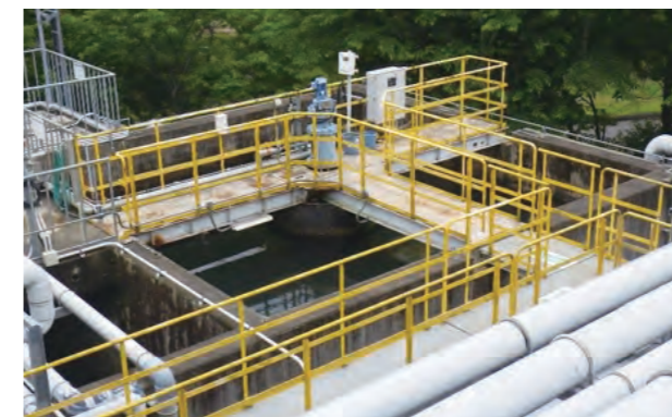
Wastewater treatment facility
